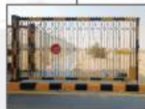
A1 Auxiliary Gate
