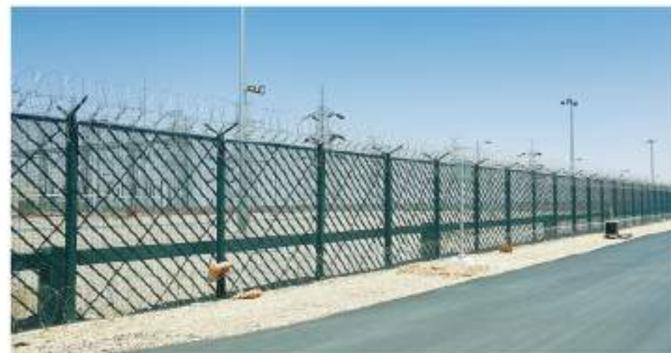
380kv substation, Sudair
