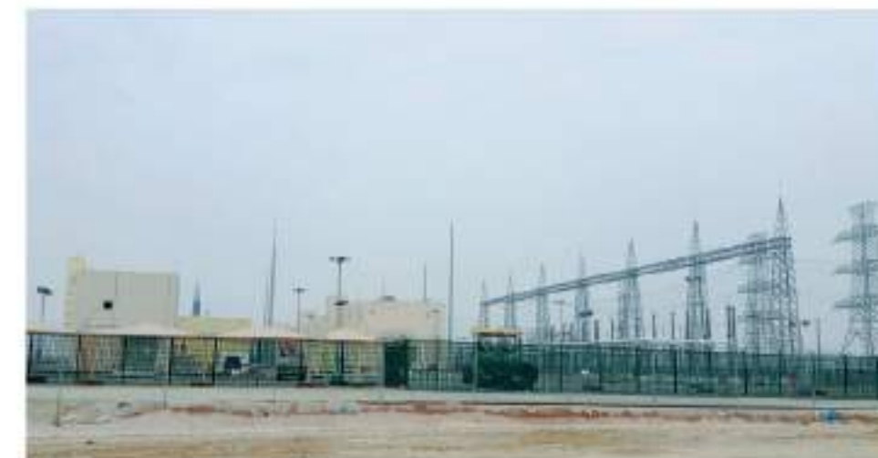
SEC 380kv Substation, Marjan, Tanajib
